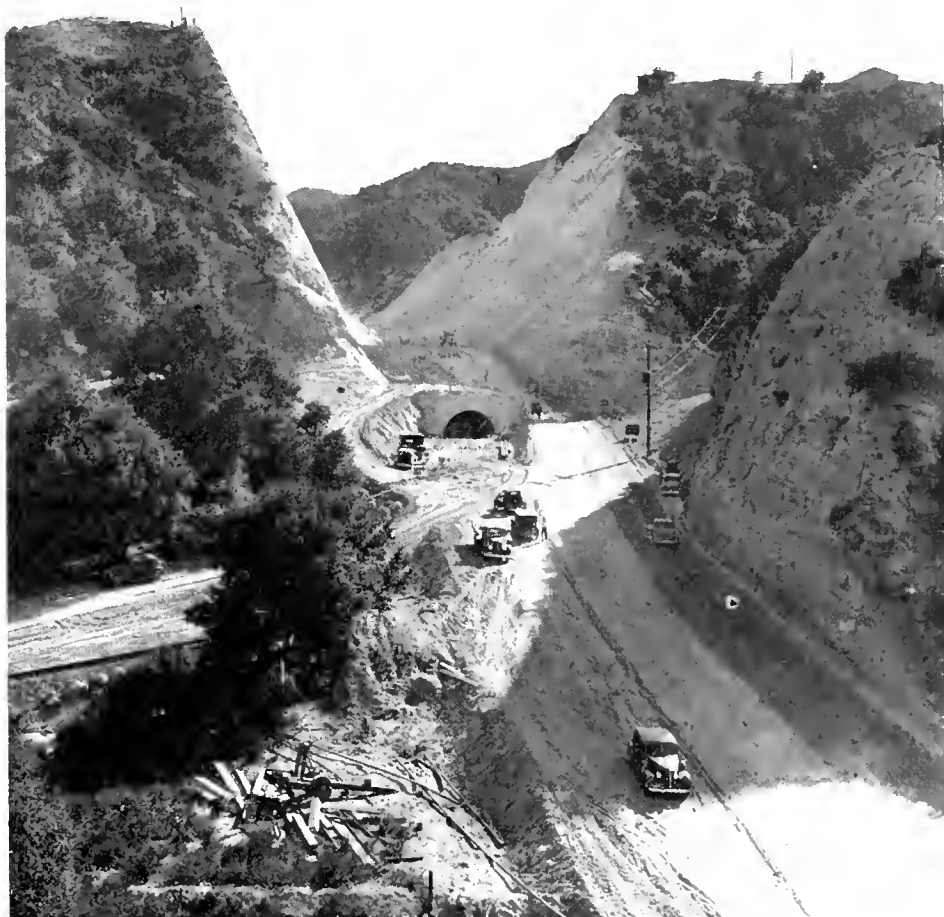
Newhall Tunnel, cut through the Santa Susana Mountain ridge in 1910, is shown as it appeared in 1940, while in the process of being transformed into an open cut highway
